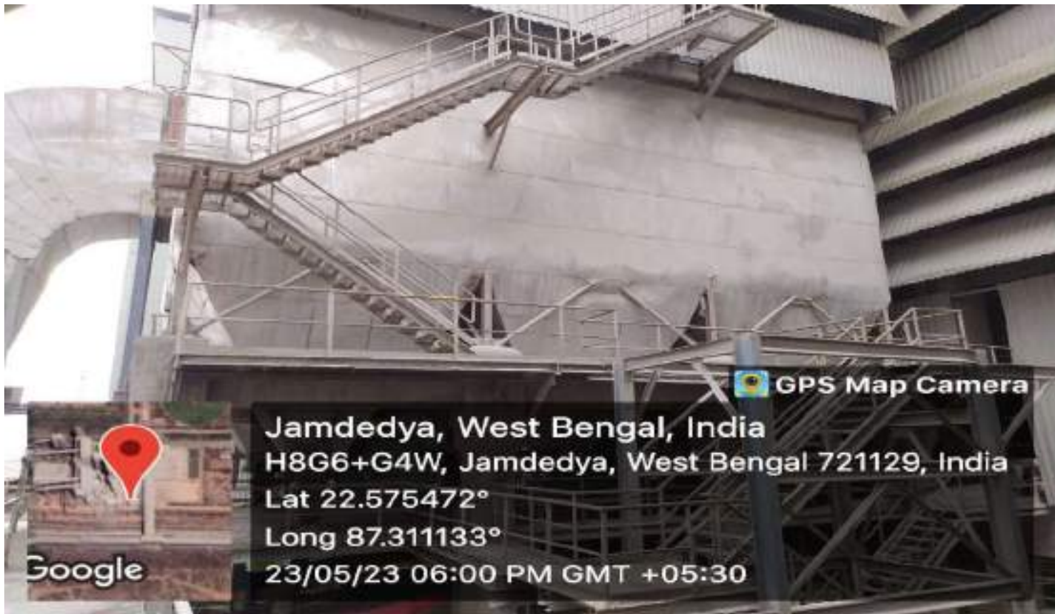
High Efficiency Bag Houses attached to grinding circuit(Photograph - I)
