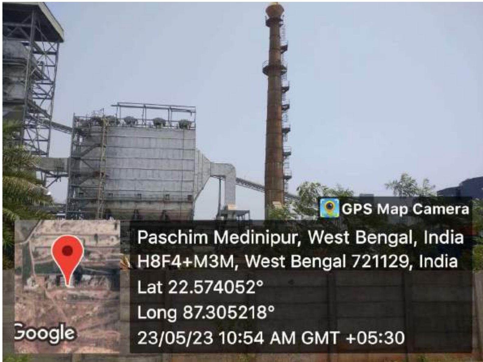
High Efficiency ESP installed after the boiler(Photograph - II)
