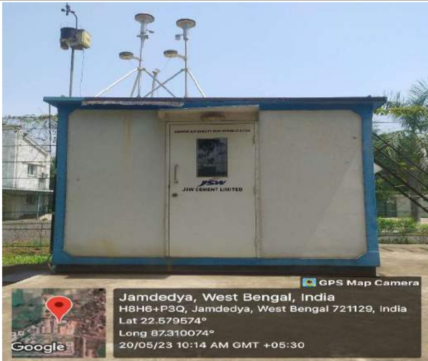
Continuous Ambient Air Monitoring Station (Photograph - III)
