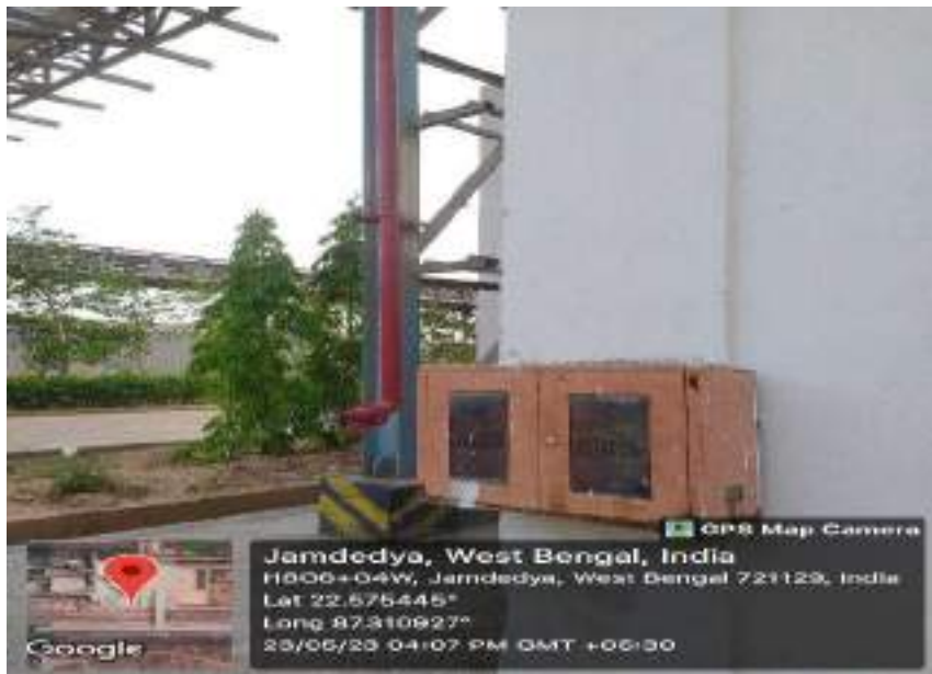
Fire Fighting System (Photograph-XXX)
