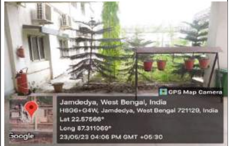
Fire Fighting System (Photograph-XXXIII)
