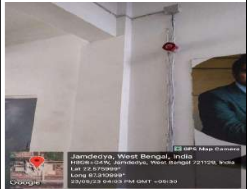
Fire Alarm (Photograph-XXXI)
