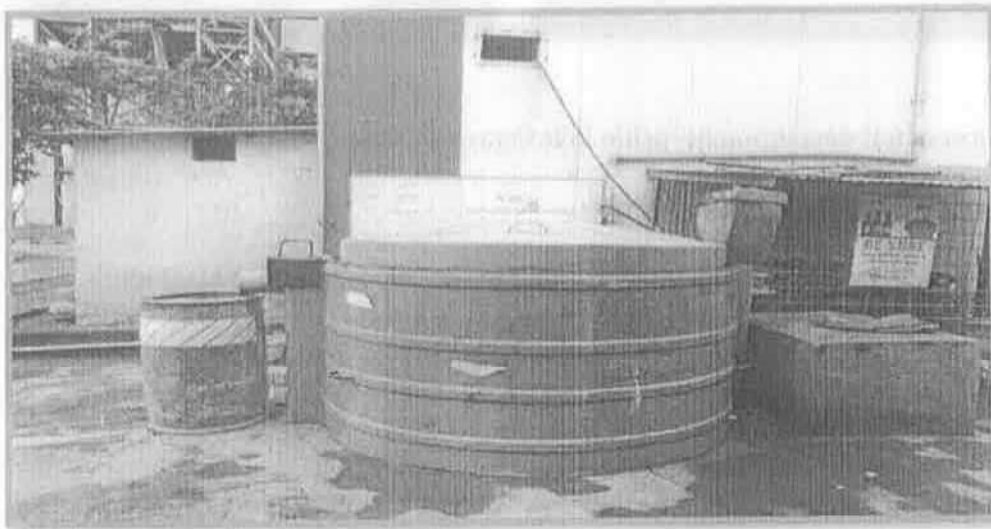
Bio gas plant installed at near canteen
