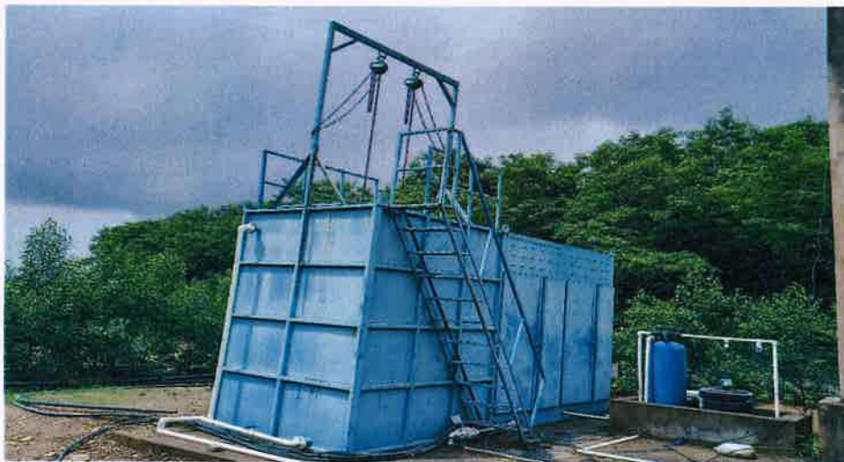
20 KLD Sewage Treatment Plant installed for treatment of domestic water
