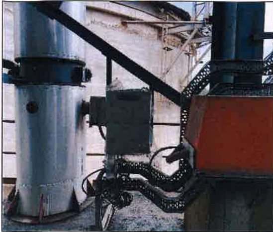
CEMS installed for Coal Mill
