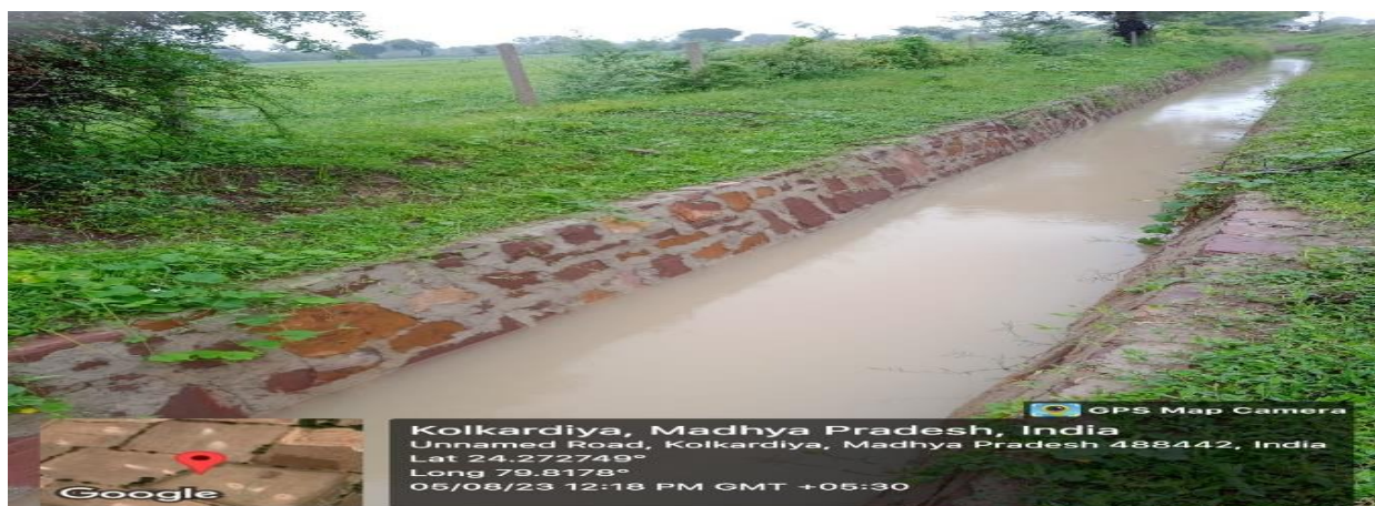
Rainwater Harvesting in Garland Drain
