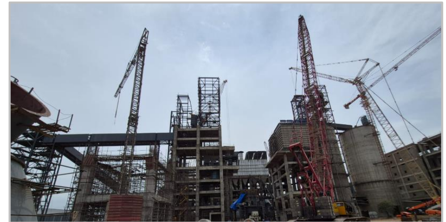
Nagaur IU – Cement Grinding and Packing & Dispatch
