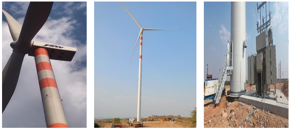
Wind capacity at Vijayanagar plant
