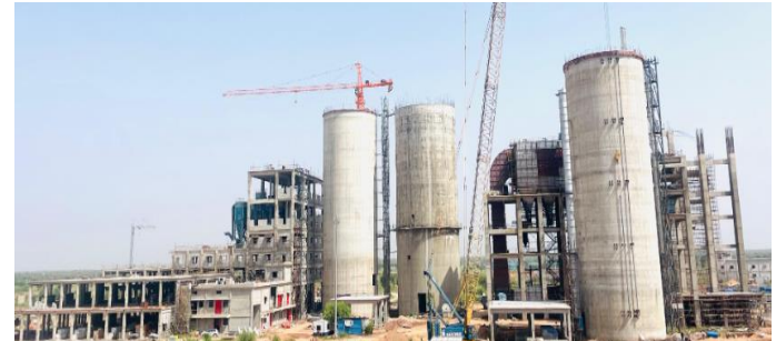
Nagaur IU – cement grinding and packing & dispatch
